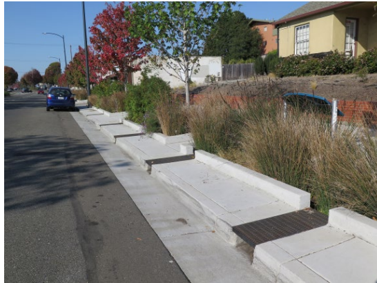
Curb cuts directing water to planting areas
