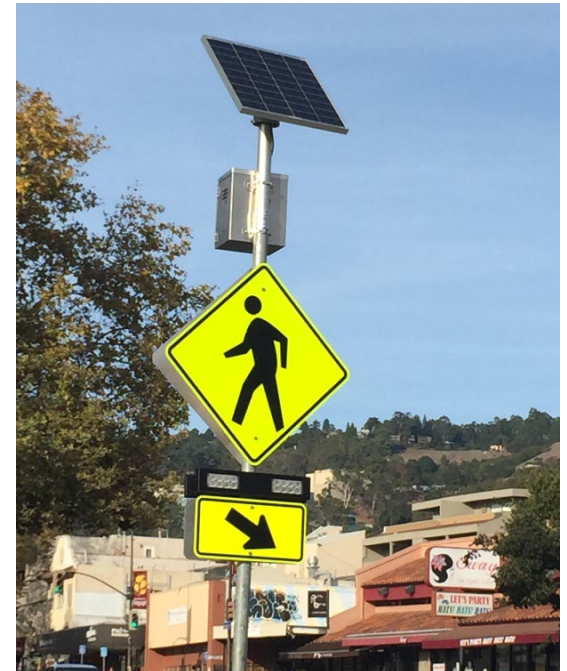
Solar-powered pedestrian signal
